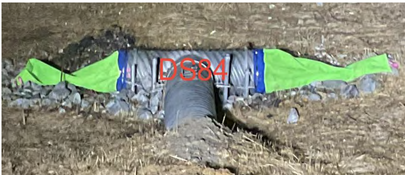
California Department of Transportation (CALTRANS) Installation
