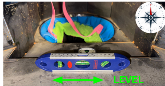
Interface Funnel and filter hanger are level from East to West (Front View)
