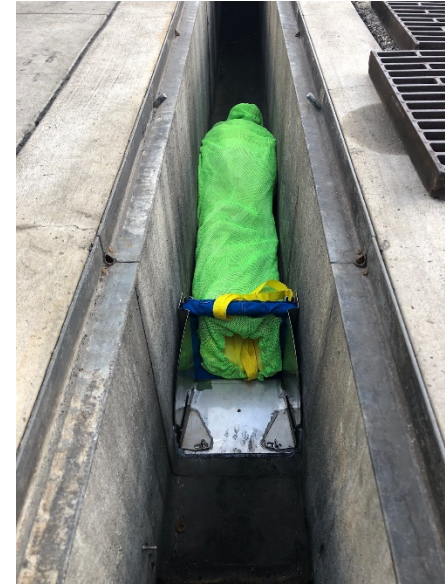
Channel Filter System (CFS)
